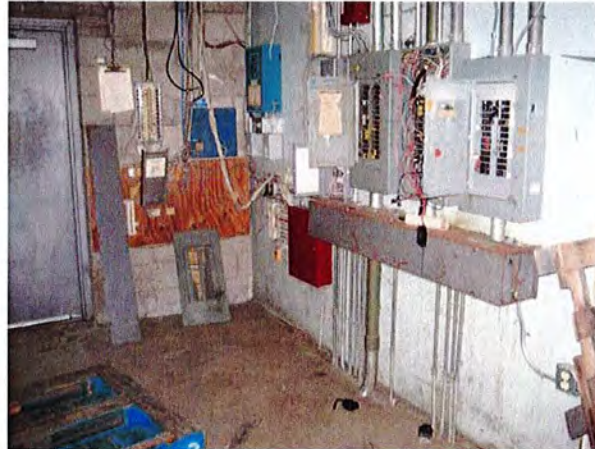
Utility room within subject property building.
