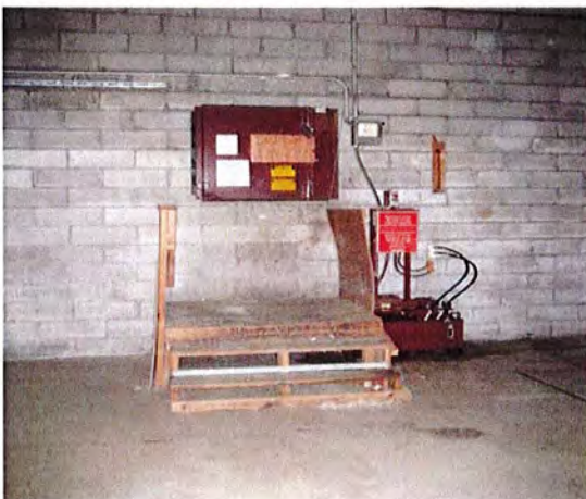
View of trash compactor unit in rear of subject property building.
