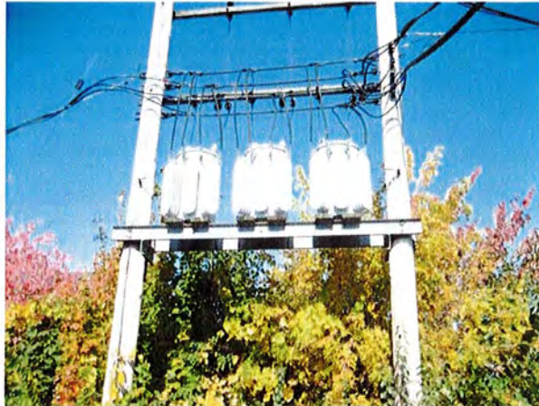
Pole-mounted transformers located immediately to the north of the subject property building.
